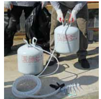
Shaking of A-side and B-side tanks
